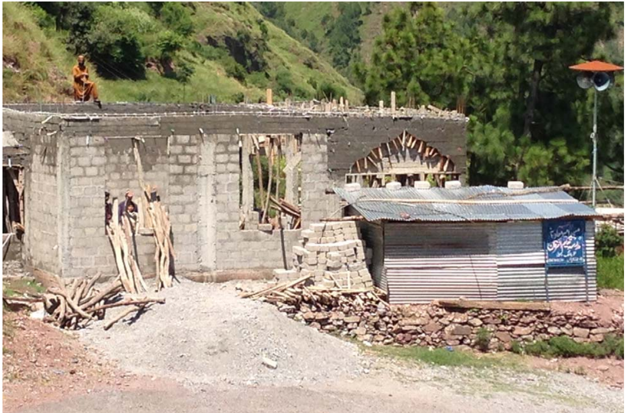
Ten years after the earthquake, a family in Balakot starts constructing the house, after receiving money from a family member who works in the Middle East.
