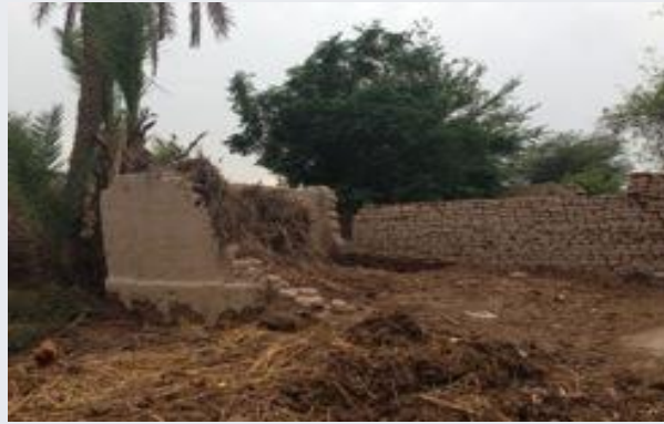
Destruction brought on by floods 2010 is still evident in the village
