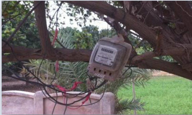
Lukwala: Electricity meter fixed on a tree by electricity department has created risks
